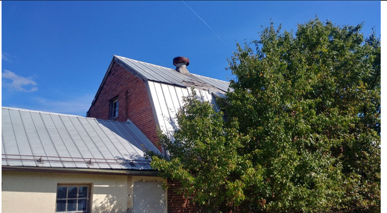
Exterior Roof – Damaged To Be Replaced
