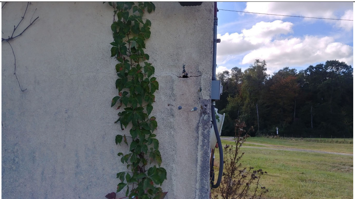
Exterior Masonry – Crack Shows Damaged To Be Repaired
